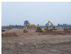
Site work at FDMCH Crescent Woods, a new RCI neighborhood on Fort Drum
